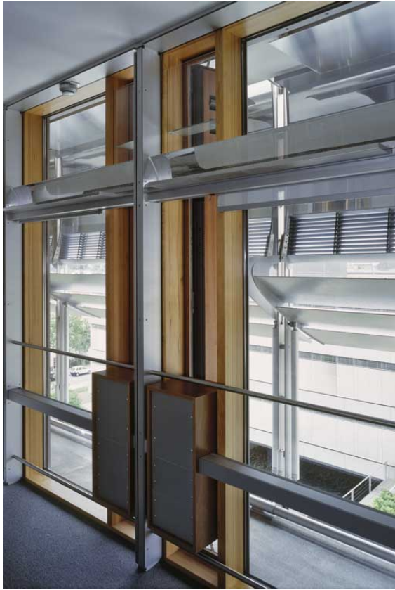
Inner façade, integrated installations
